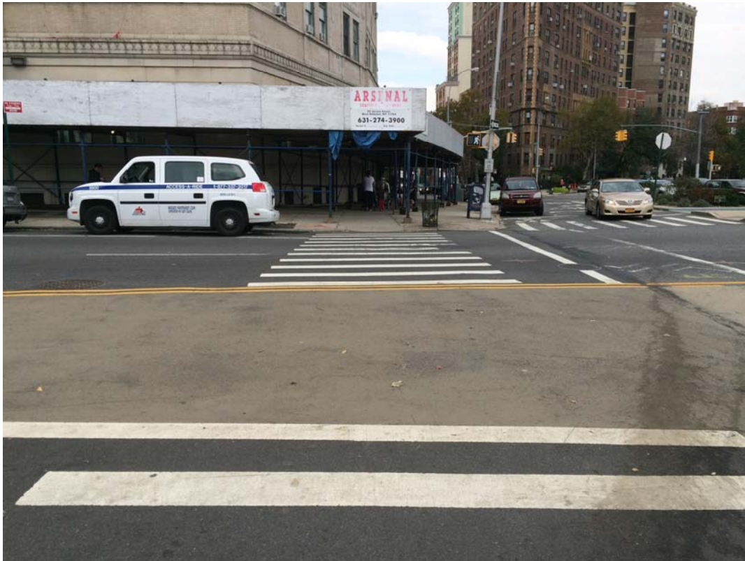
Figure 5. Painted pedestrian plaza without detectable warning strip at crosswalk (Grand Army Plaza, Brooklyn)
