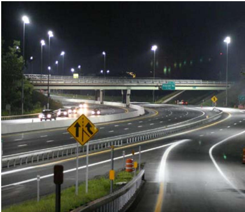
High-mast Work Zone Lighting Photo by Dennis Guyon
